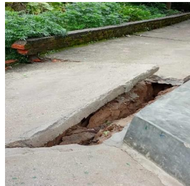
Damage at Sathya Uddhyan
